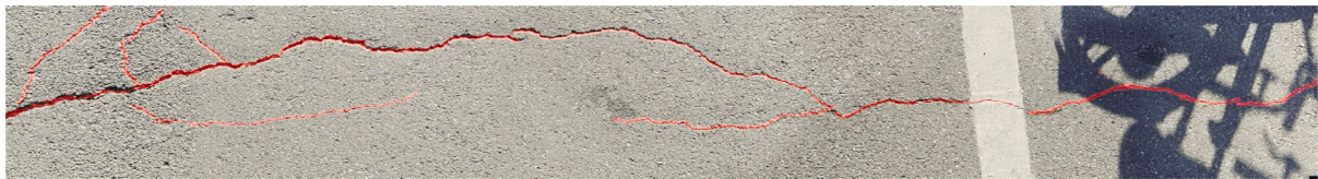
(e) Sample 3: asphalt, strong lighting, transverse crack, with markings
