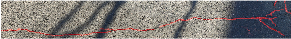
(c) Sample 5: asphalt, mottled, longitudinal crack
