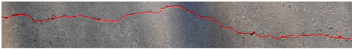
(a) Sample 11: concrete, mottled, longitudinal penetrating crack
